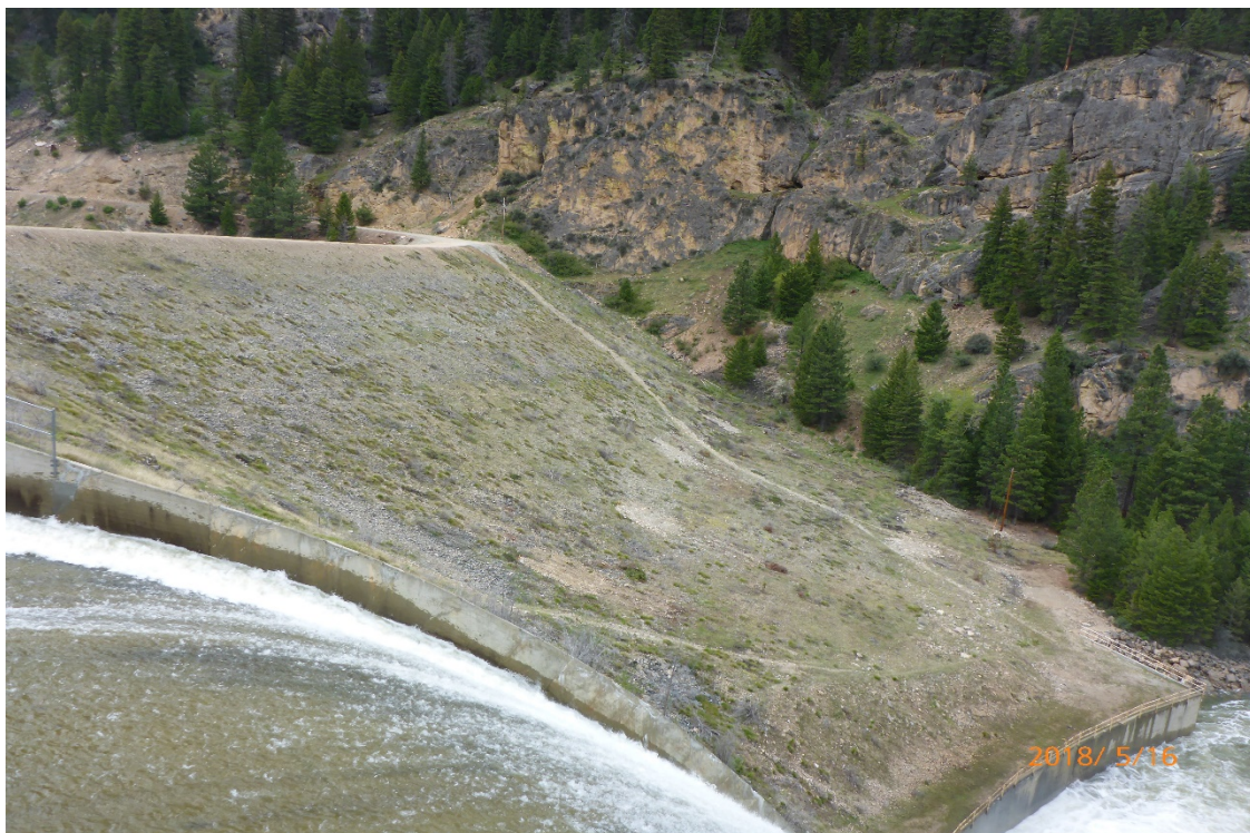
Tow area of Painted Rocks Dam, currently inaccessible by vehicle without fording river.
