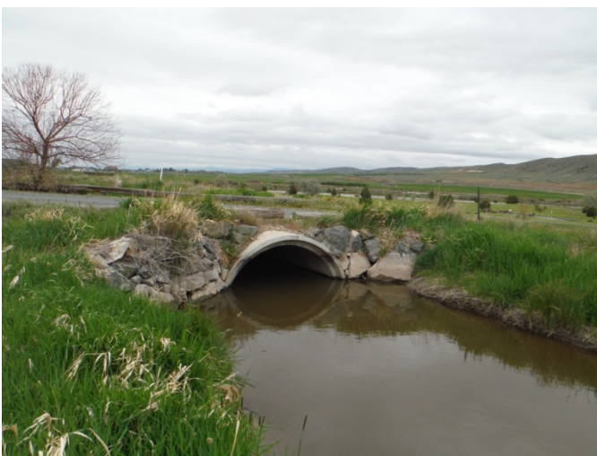
Undersized culvert at access point
