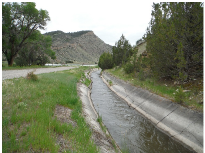
Concrete lined section of West Canal, with lining failure.
