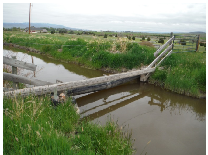
Improperly designed/constructed fence crossing
