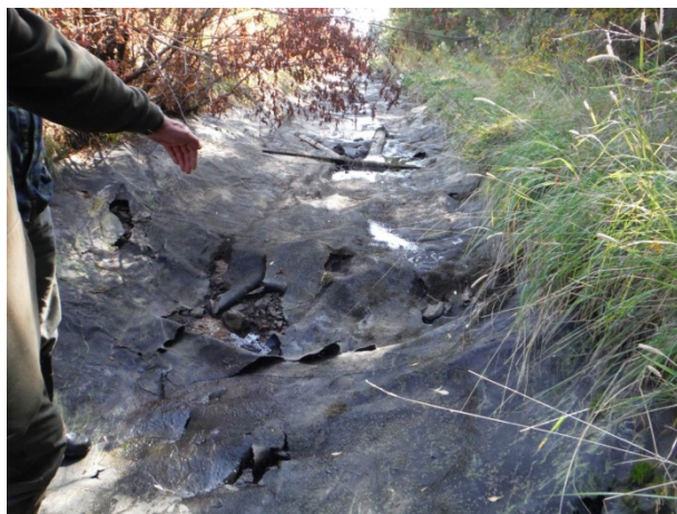
Existing Damaged Liner
